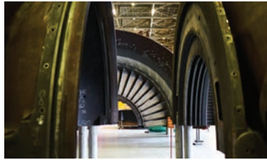
Far left: The Darlington turbine hall. For the first time all turbine blades and rotors were removed and reinstalled to ensure continued operation for another 30 years
