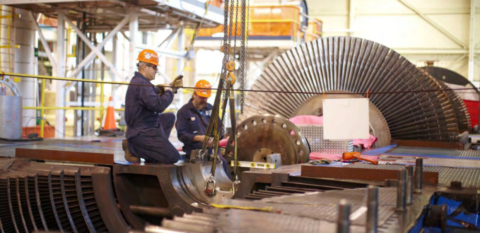
Workers at Ontario Power Generation's (OPG) Pickering Nuclear during a planned maintenance outage. Image: OPG
